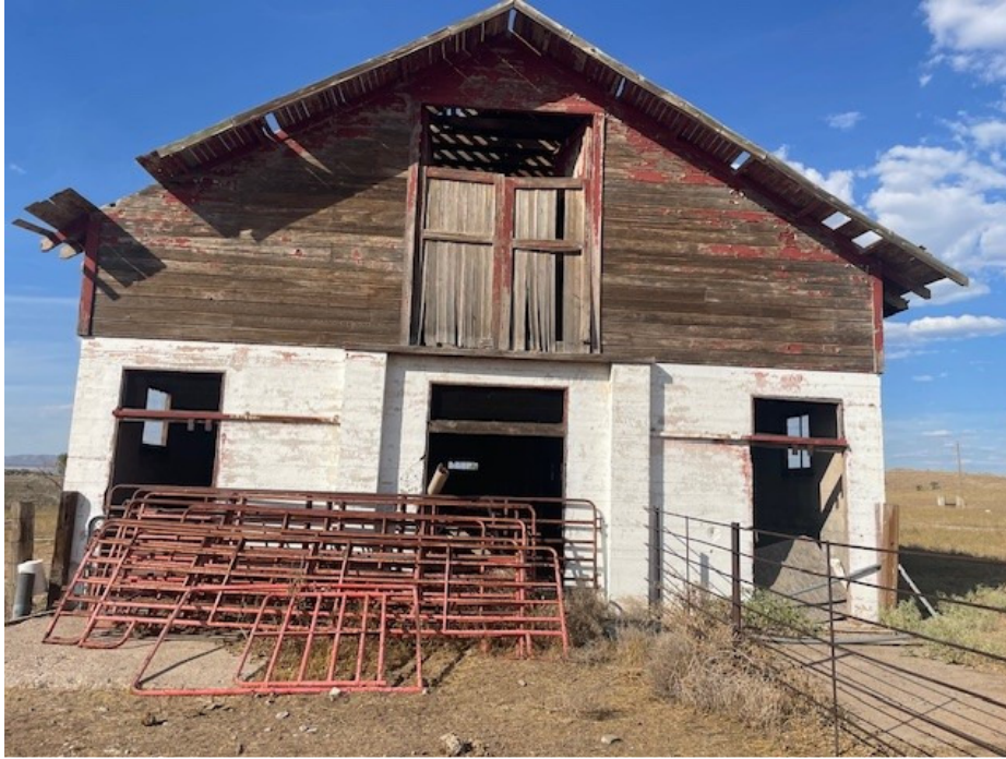
South elevation showing required soffit repairs & missing doors. Upper hay Loft doors to be covered with OSB panels.
