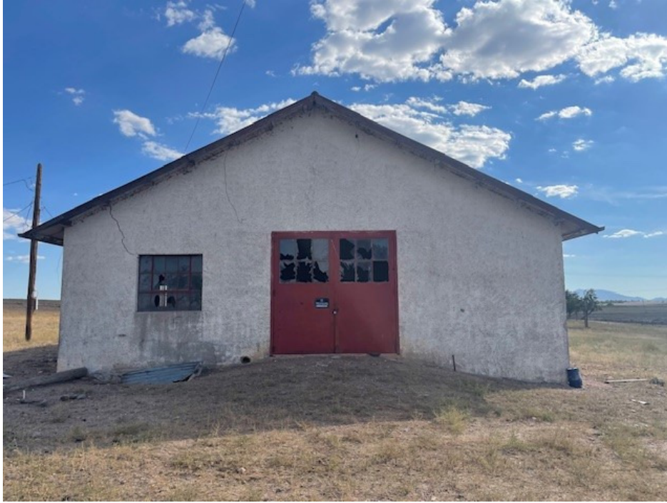
North elevation, replace glazing, repair crack at northeast corner.
