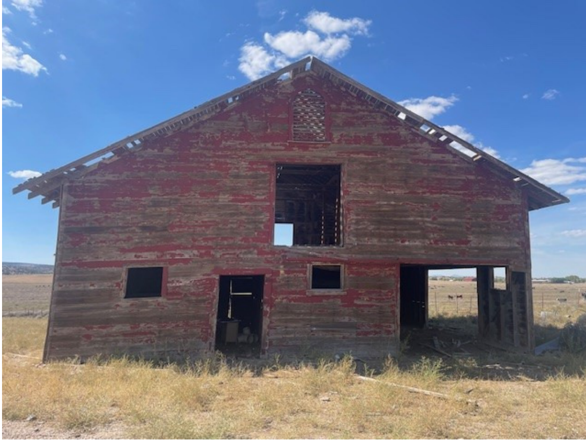
East elevation, south wall leaning. No foundation, earth to wood contact.
