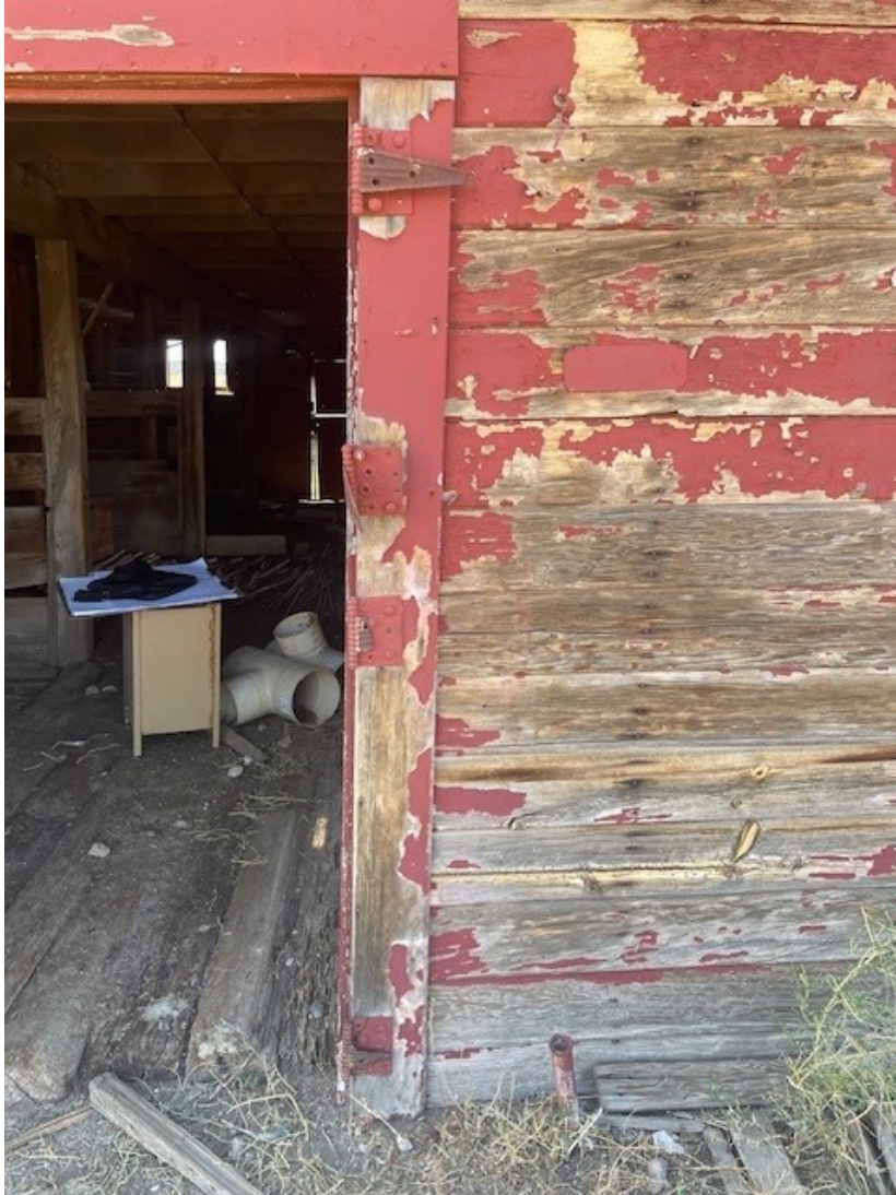
Exterior door. Railroad tie floor, may contain toxic materials.
