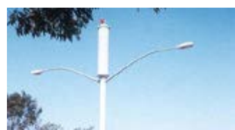
▣ Figure 7 Antennae on Parking Light Stand
