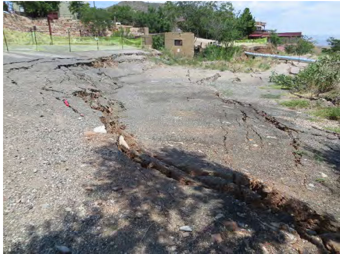
Figure 70 Photo of Jerome Landslide Related Damage
